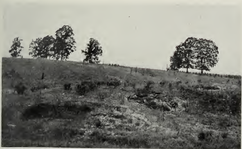
FIG. 17.—Side-hill breaks near Cuba caused by room-and-pillar mining of a 5-foot bed of coal from 50 to 75 feet deep.
